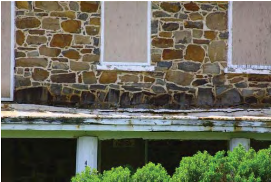
Deterioration Of Front Porch Roof Framing
