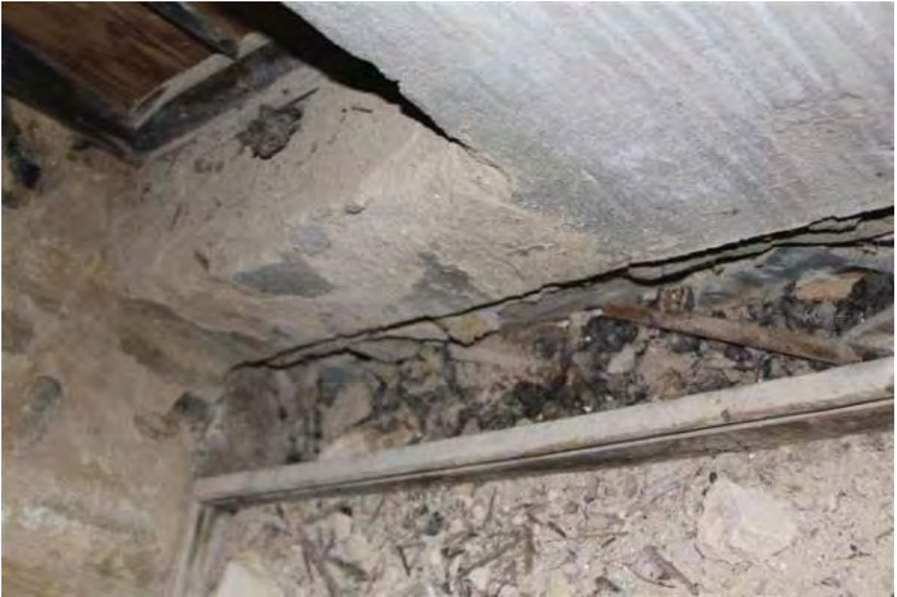
Wall Displacement At Left Side Wall
