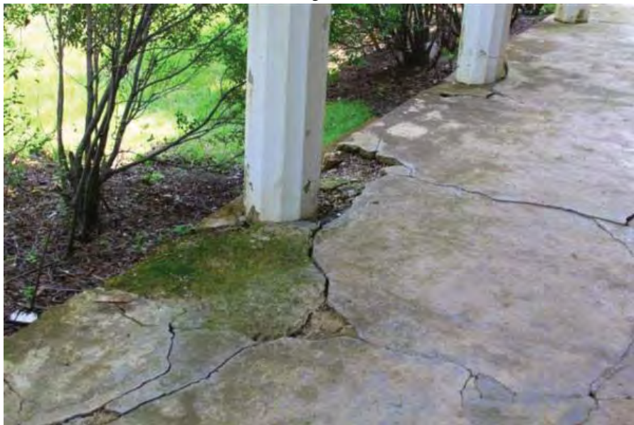
Cracks And Settlement In Front Porch Slab At Concrete Columns
