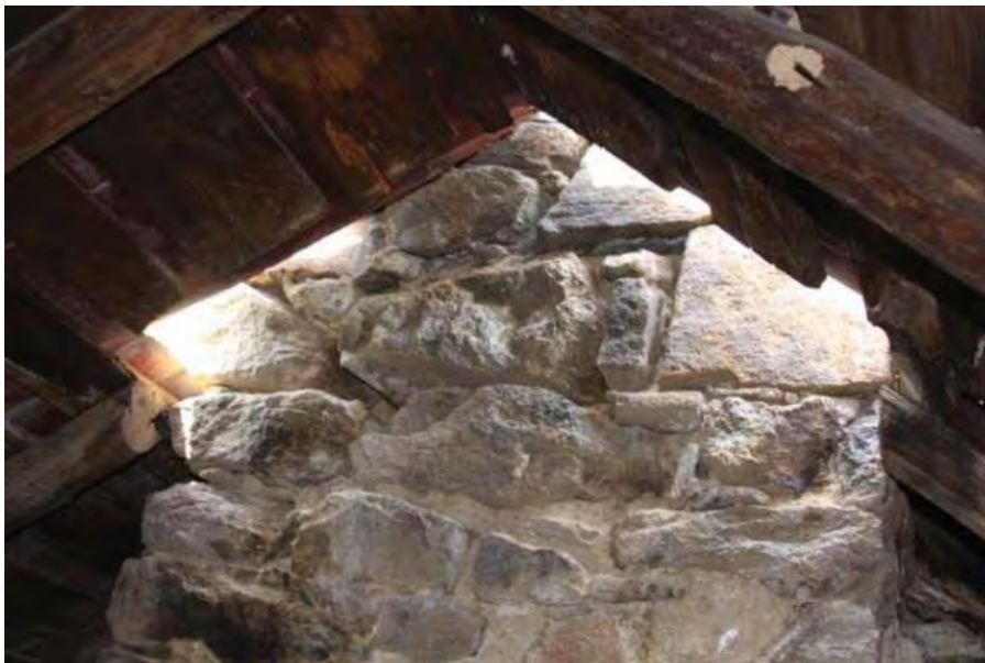
Gap Between Roof And Chimney – Right Side
