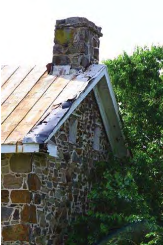
Chimney Displacement On Right Side Of House
