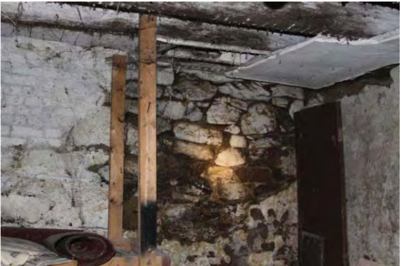
Water Damage In North West Corner Of Basement
