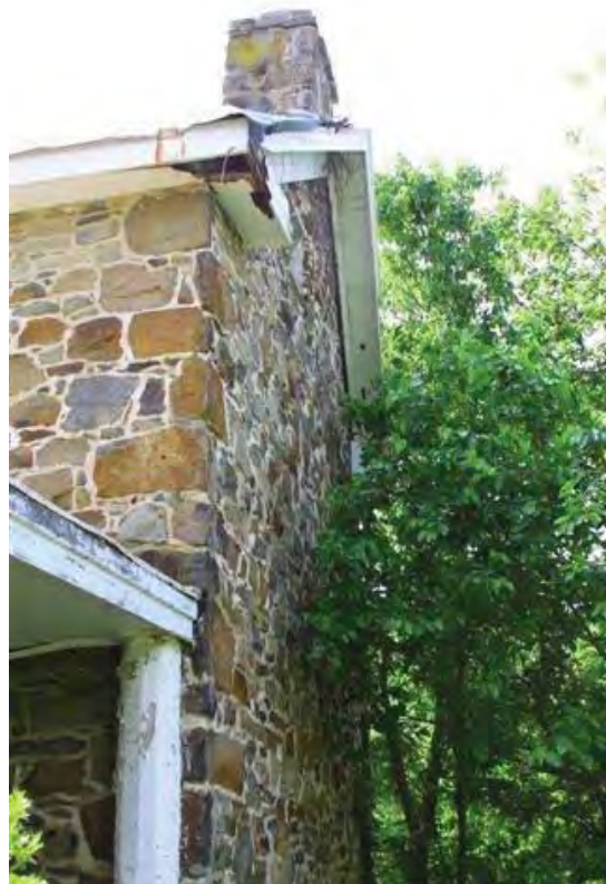
Right Side Elevation And Chimney And Wall Displacement
