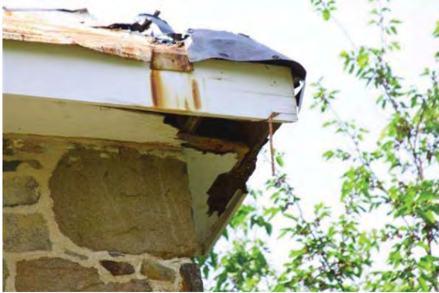
Water Damage And Rotting Wood At Roof Eave
