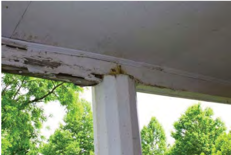
Deterioration Of Framing Members At Front Porch
